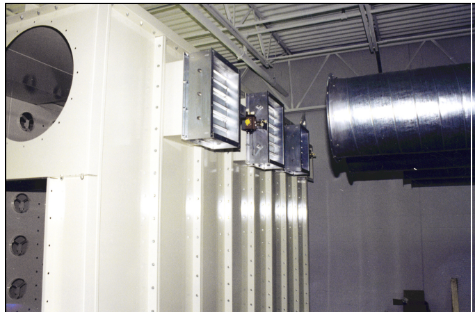
Figure 7 Ducting to an Osprey Stand Alone Final Filter.
